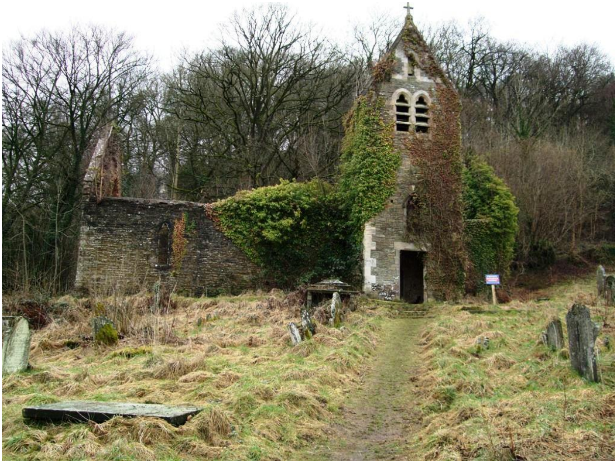
Fig.38 The picturesque, but dilapidated church of St Mary (many fine features such as the tracery east window are in a state of very poor repair)
