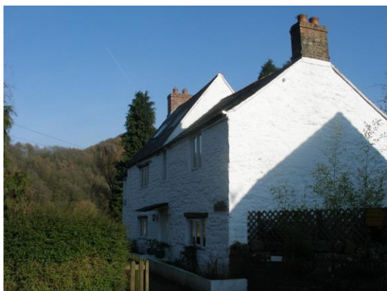
Fig.54 Quay Cottage faces the river. The simplicity of cottage design and layout is apparent in this image. Walls are painted rubble.
