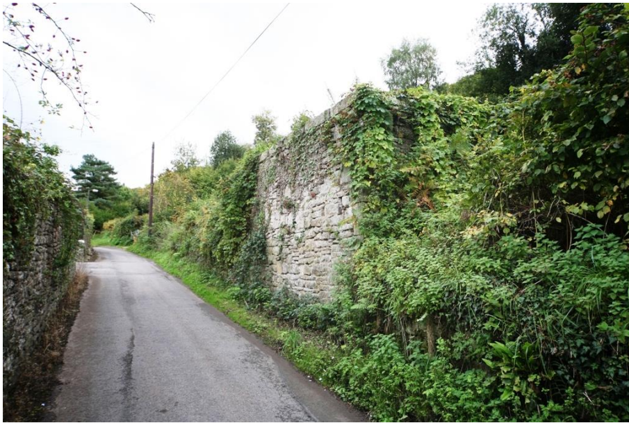
Fig.37 A dilapidated stone structure, recorded as a Pound on the first edition ordnance survey map
