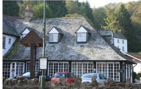
Fig.33 A well executed traditionally laid roof of diminishing slates at the Royal George Hotel
